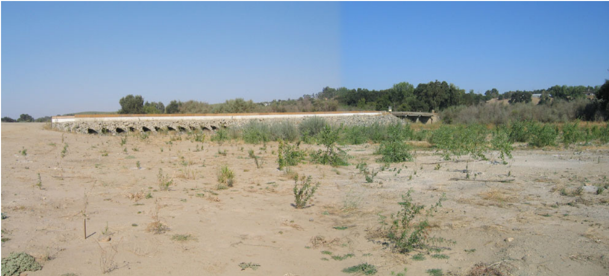
Figure 60. Series of twelve culverts in 7/11 Reach that bypasses high flows on the floodplain through the southern abutment of the 7/11 Materials haul road bridge.
